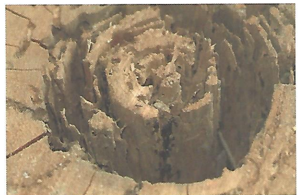
Carpenter ant galleries in wood.
